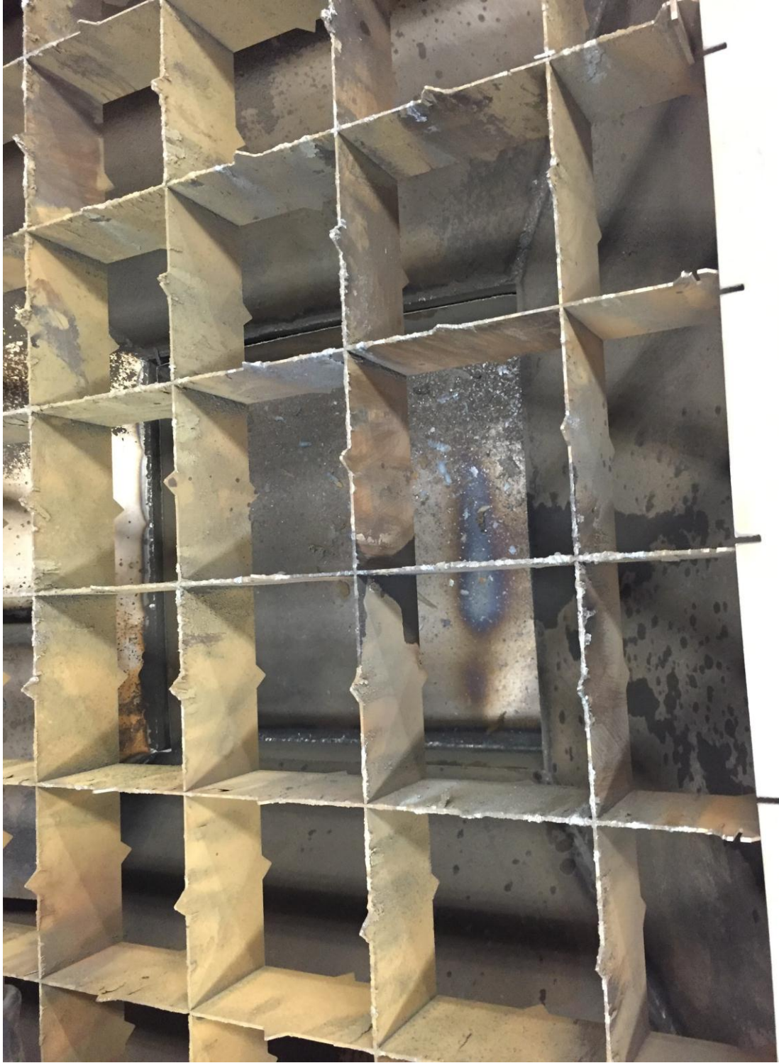
The freshly cleaned PlasmaCam ventilation system.
